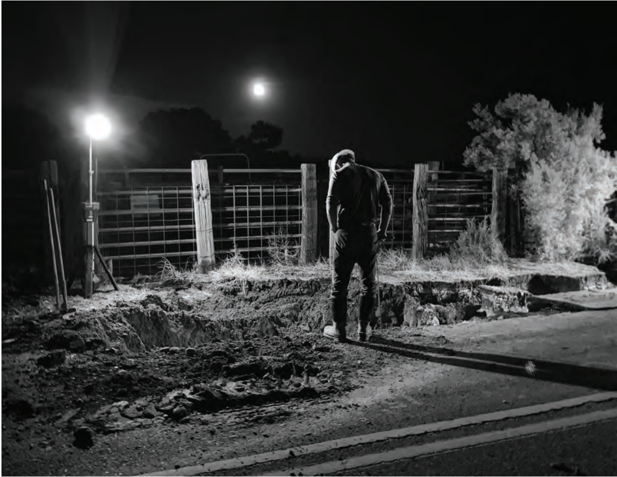
Above Photo by Andrea Lopez - Engineering Technician, Braden Box, assesses a leak in the Redlands area.
